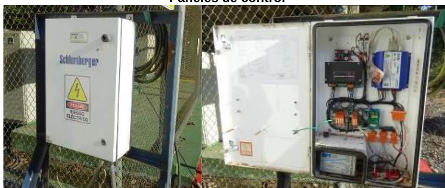
Paneles de control
